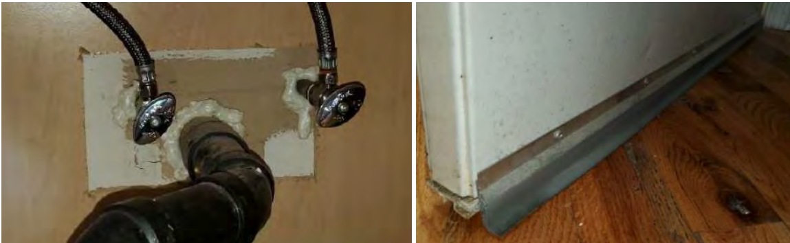
Figure 8. Example of spray foam air sealing around kitchen pipe penetrations (left) and screwed-on door sweep (right)
