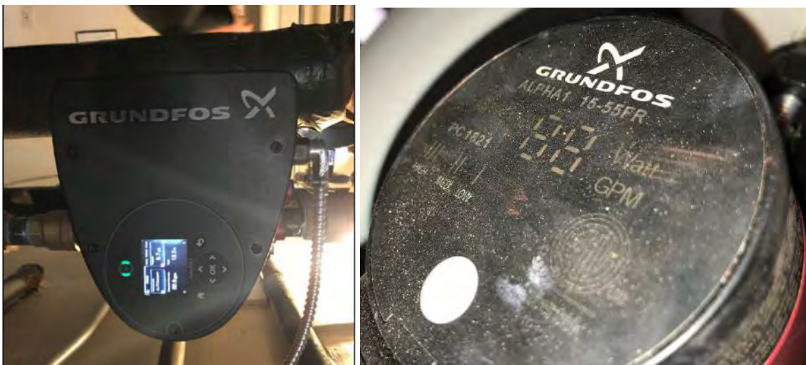
Figure 10. Example of installed ECM pumps
