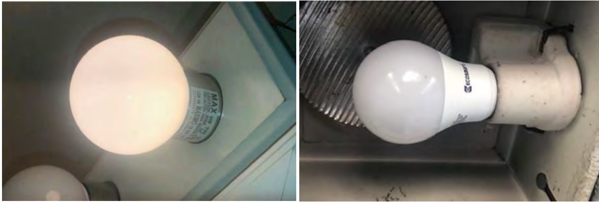
Figure 4. Example of LED bulbs installed in dwelling units
