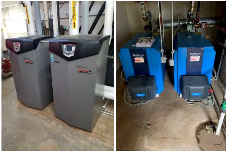
Figure 13. Examples of installed condensing boilers
