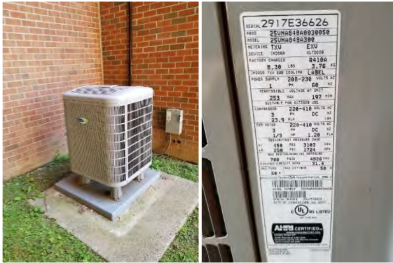
Figure 12. Example of installed heat pump outdoor unit and nameplate
