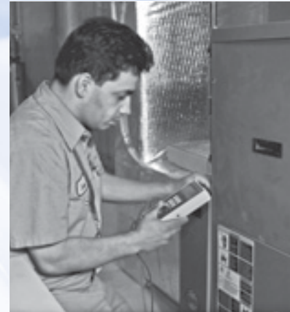
Ensuring proper ventilation during the CTEHHI service.
