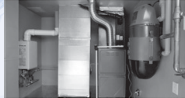
Geothermal heat pump equipment
