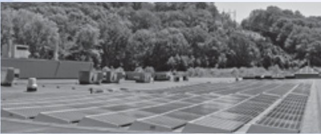
Solar photovoltaic installation
