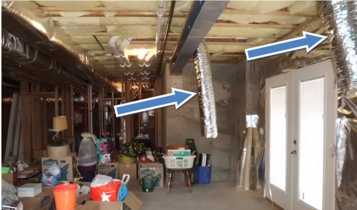
Figure 0-17: Hanging Flexible Ducts Serving as Pressure Relief
