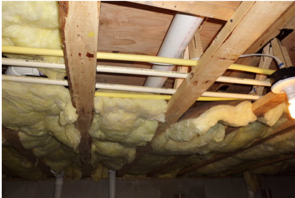
Figure 0-5: Poorly Installed Frame Floor Insulation
