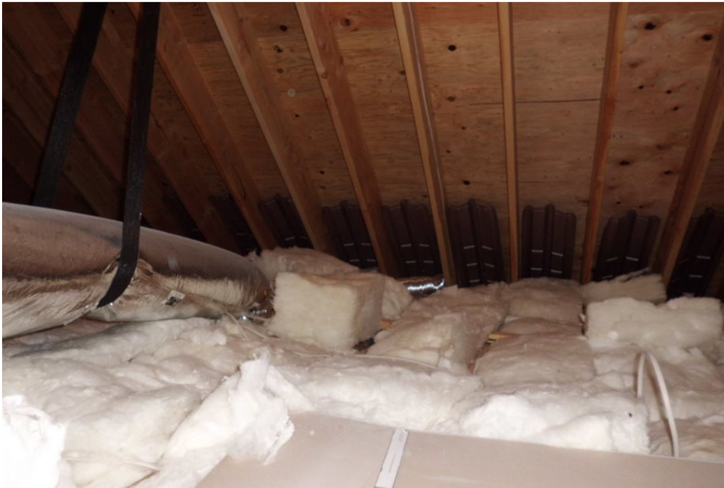
Figure 0-10: Poorly Installed Fiberglass Batt Attic Insulation
