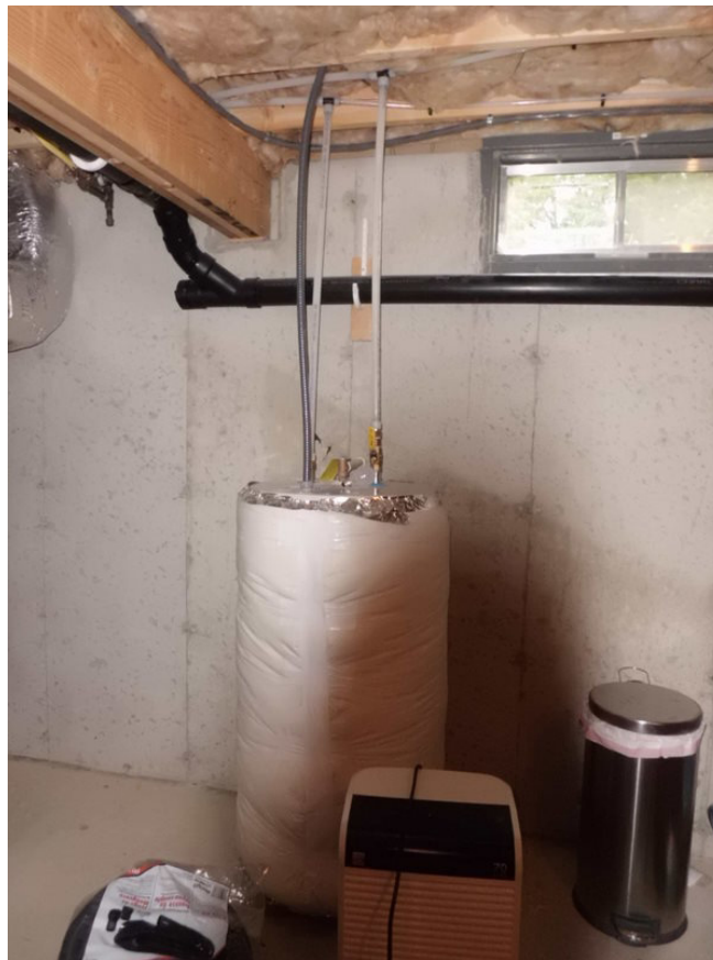
Figure 0-15: Insulated Indirect Water Heater
