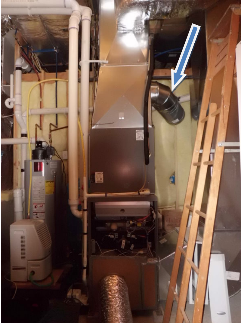
Figure 0-16: Pressure Relief Diverter & Uninsulated Supply and Return Ducts
