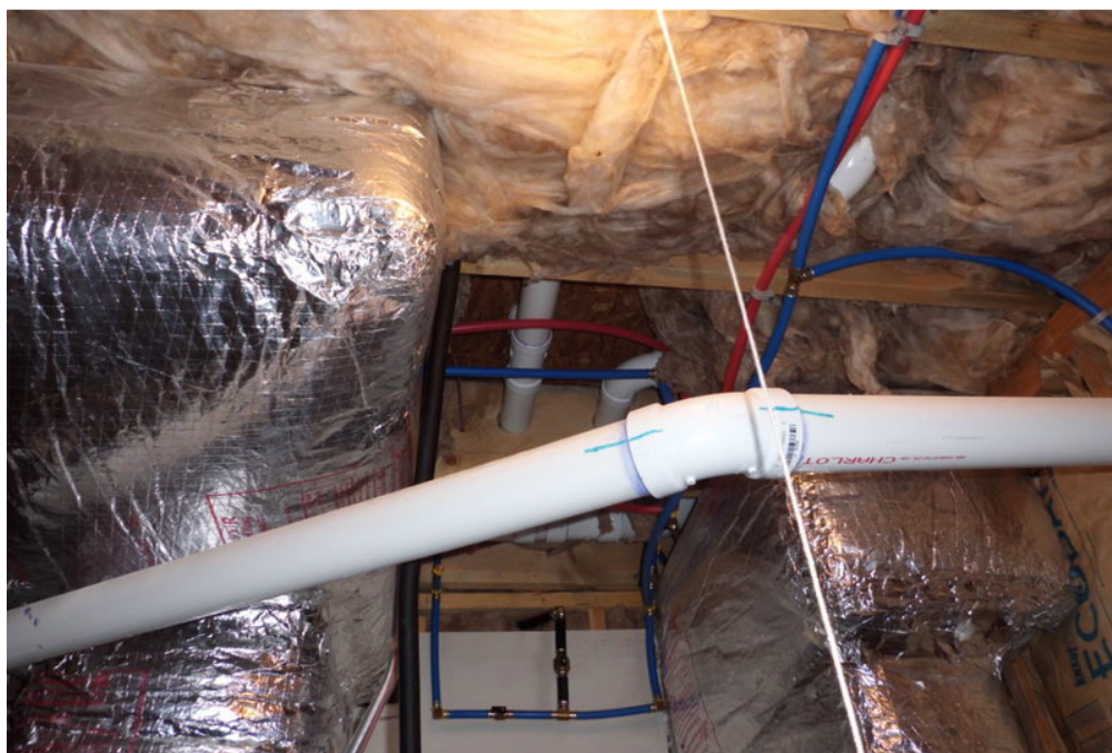
Figure 0-6: Gaps in Frame Floor Insulation and Uninsulated DHW Lines
