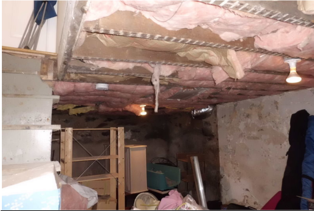
Figure 0-4: Poorly Installed Frame Floor Insulation
