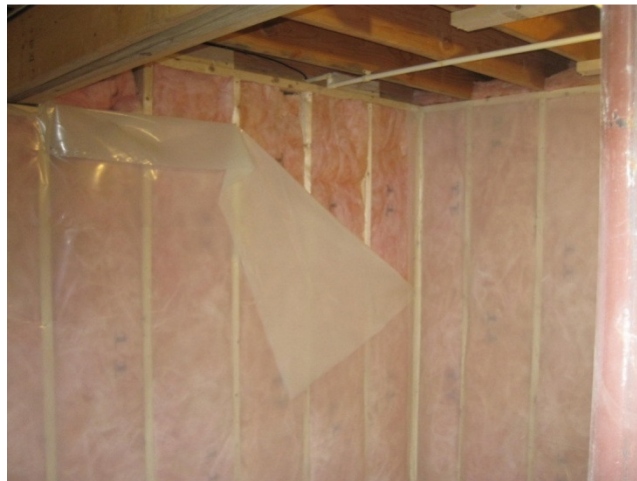
Figure 0-2: Grade II Fiberglass Batts—Basement Walls
