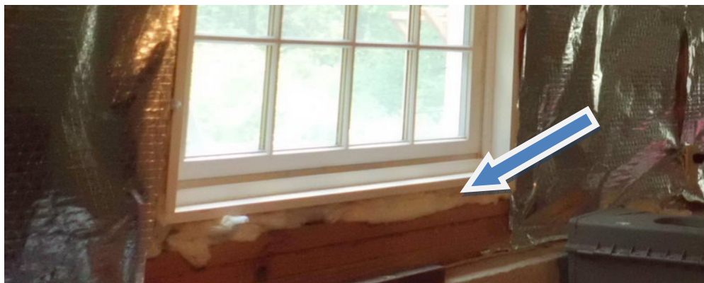
Figure 0-12: Fiberglass as Ineffective Air Sealing
