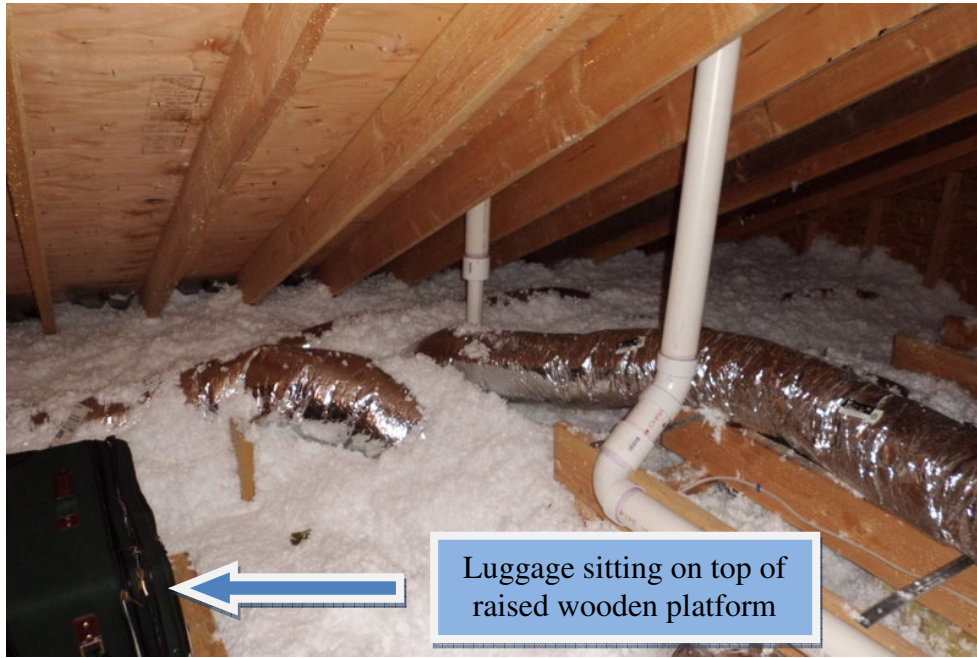
Figure 0-11: Blown-in Fiberglass Attic Insulation with Storage Platform
