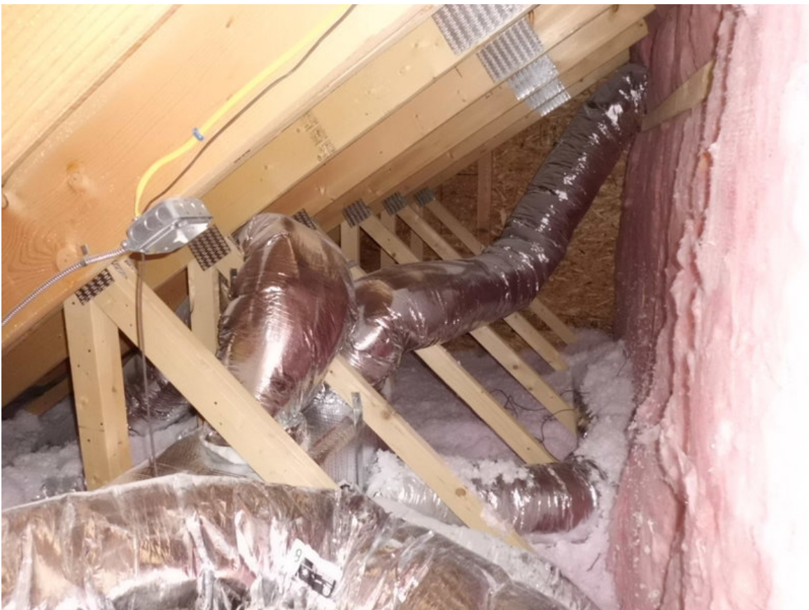
Figure 0-14: Kinked Ducts Exposed to Wind-Washing behind Knee Wall
