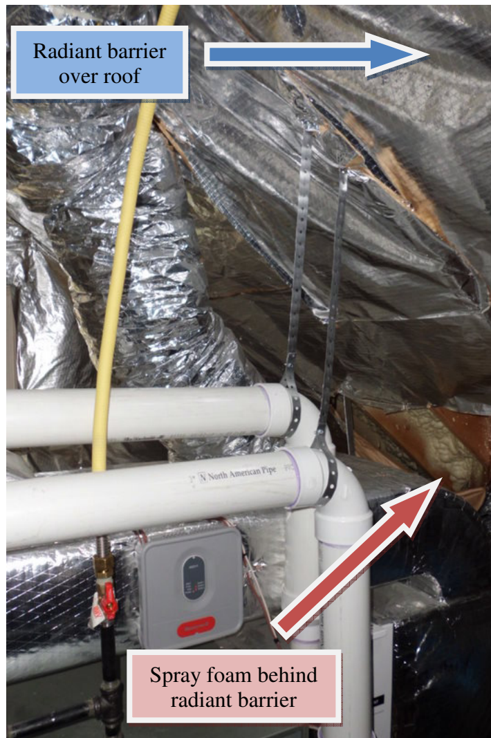
Figure 0-13: HVAC System in Conditioned Attic
