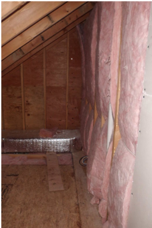
Figure 0-9: Poorly Installed Fiberglass Wall Insulation
