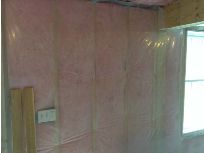
Figure 25: Grade II Fiberglass Batts—Basement Walls
