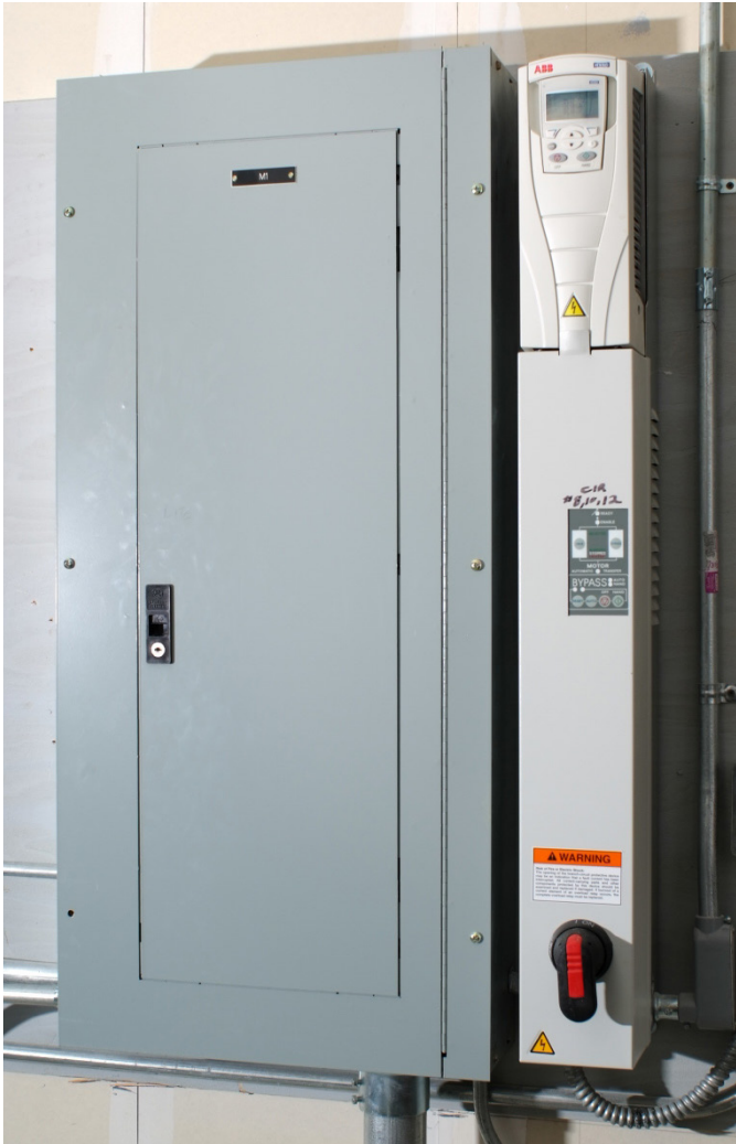
VARIABLE FREQUENCY DRIVE CONTROLS ON GROUND-WATER SOURCE HEAT PUMPS REDUCE ELECTRICITY USE.
