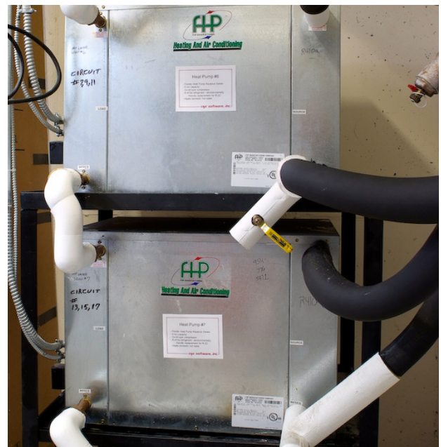
GEOTHERMAL HEAT PUMPS IN THE ADDITION, LIKE THE MAIN BUILDING, ARE A KEY PIECE OF CNC'S ONGOING EFFORTS TO REDUCE ENERGY CONSUMPTION.
