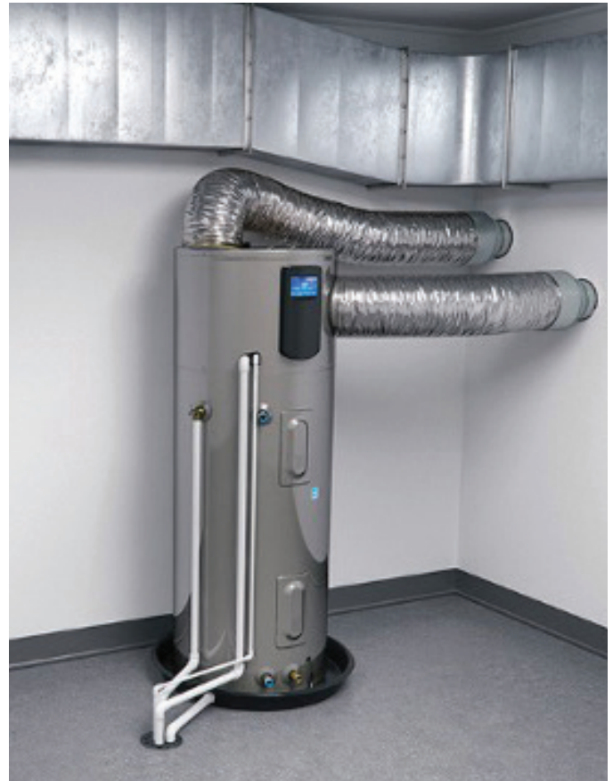
Heat pump water heater ductwork for air intake and exhaust
