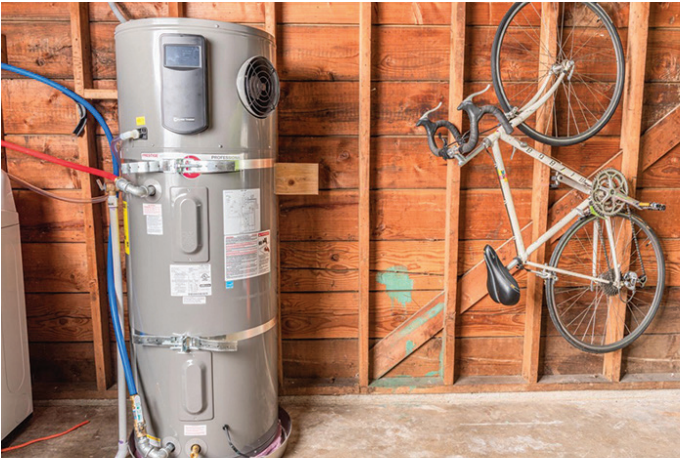
Heat Pump Water Heater
